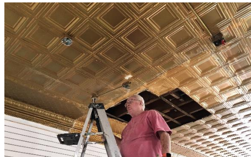
Figure 4 Mike Taking Down old Ceiling Conduit. New wiring will be installed along with 4 rows of track lights.
