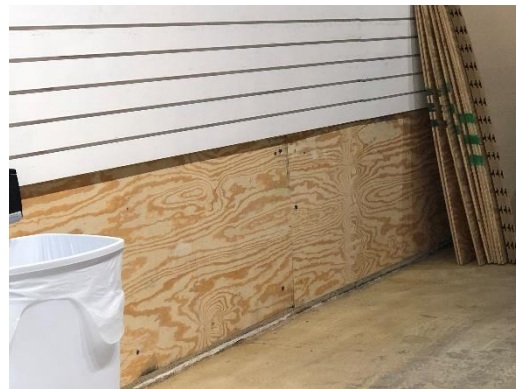
Figure 11 Plywood Installed Below Slat Wall. Conduit Will be Reinstalled with More Outlets
