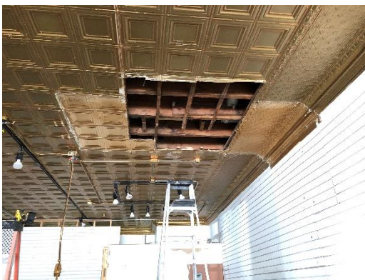
Figure 3 Hole in Ceiling from Water Leak
